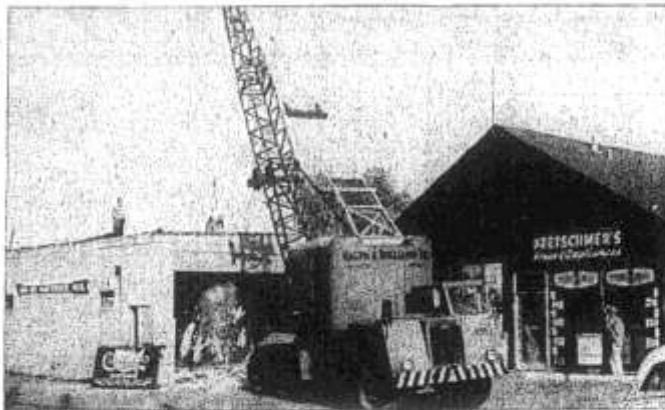
Heavy equipment clears the way for Bacon's enlarged parking lot facing St. Matthews Ave., but Kretschmer's Appliance at right has an eight-year lease, and intends to stay.
